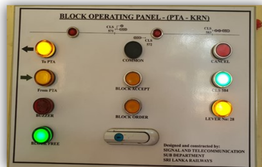
Block Operating Panel at Pothuhera
